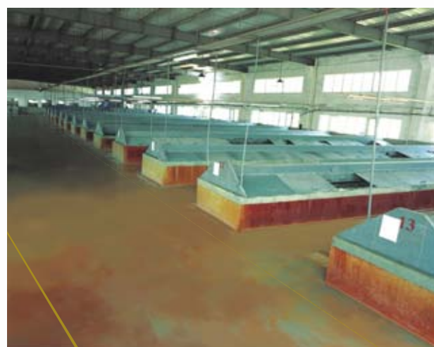
COMPUTERIZED FORMATION PLANT ◇24 formation tanks in double rows
