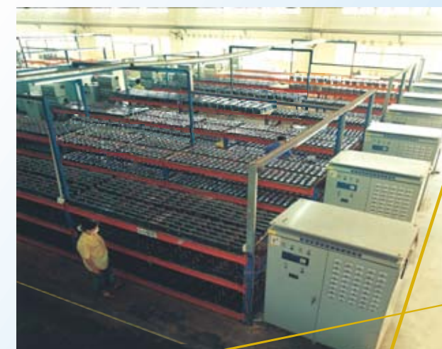
COMPUTERIZED CHARGE-DISCHARGE STATION ◇over 1800 charging circuits & over 50 chargers
